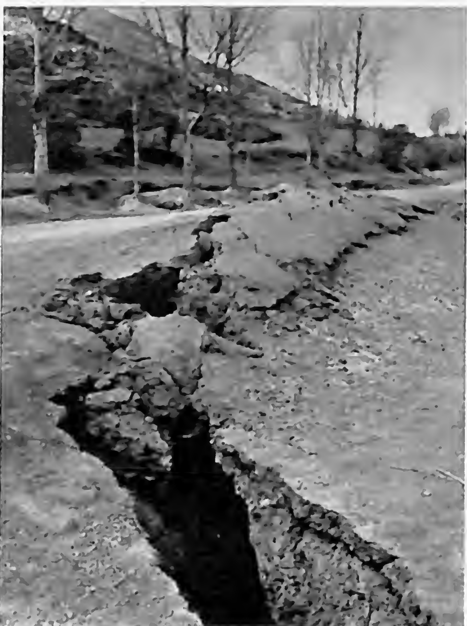
One of the fissures.
